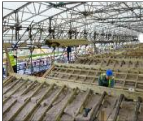
The slates have been removed from the roof, and the wool insulation is being renewed
