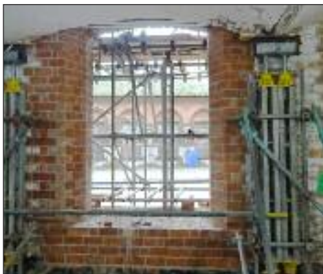
A reopened and renovated window - note the quality of the new brickwork
